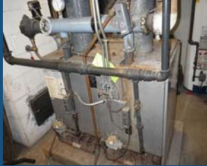
Fire Company 1 Boiler Plant
